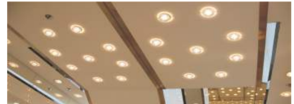
LED spot lighting
